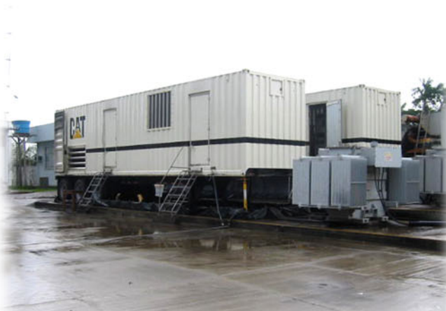
Temporary Power Modules in Iranduba, Brazil generating 3.2 MW.
