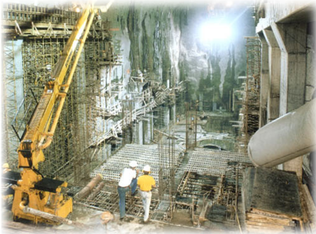
Construction for the installation of the turbines of the 375 MW La Miel hydroelectric dam in Colombia. Energy International was responsible for civil, mechanical and electrical engineering.
