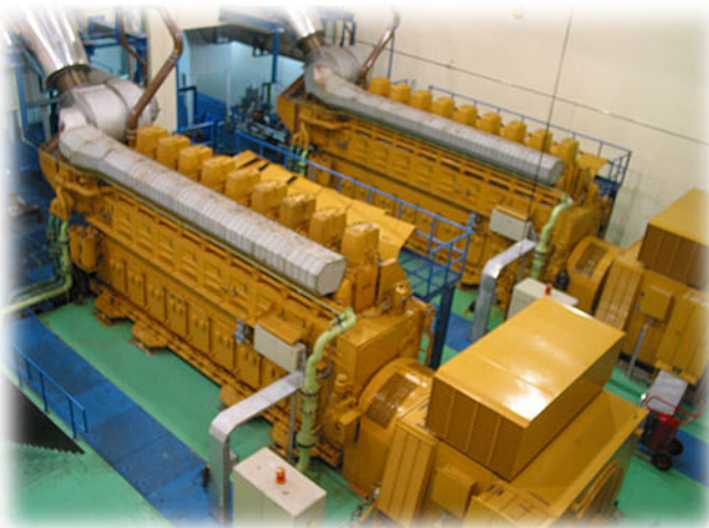
Interior of Textafil IV power plant: 2 x 9CM43 - heavy fuel oil generating 15.7 MW and cogenerating thermal oil.
