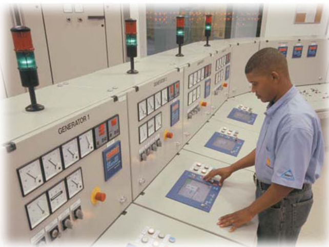
The control room at one of the power plants Energy International built and currently operates.
