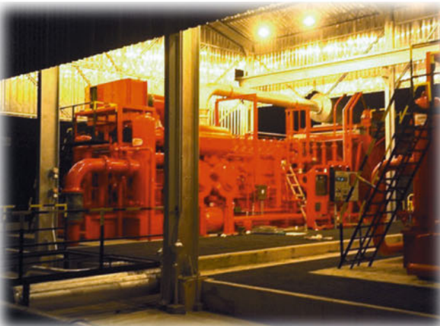
Four G3608 CAT® engines driving Dresser Rand compressors in Provincia, Colombia, at the Ecopetrol station. These compressors supply gas to the city of Bucaramanga for domestic consumption and to the refinery in Barrancabermeja.
